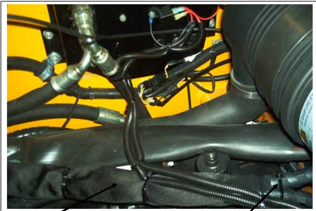
Hoses inside protective sleeve.
