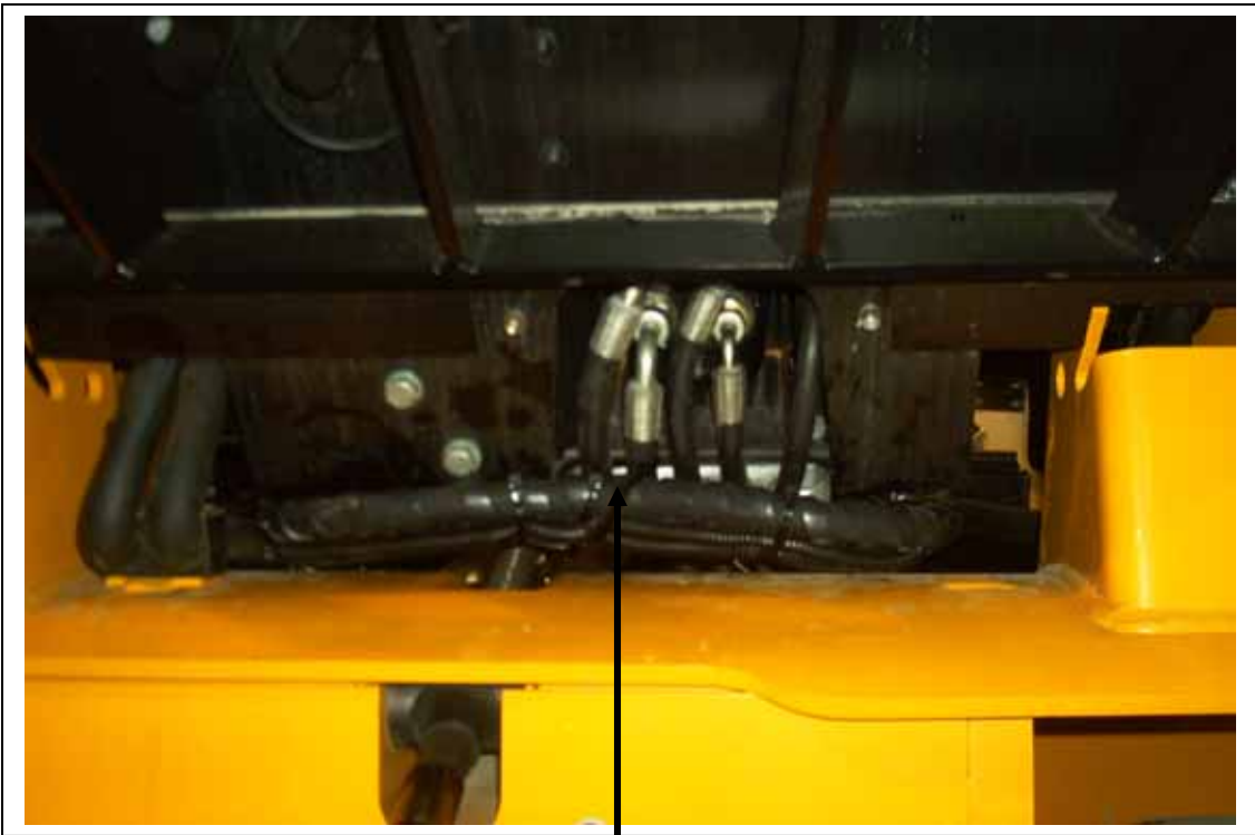
Hoses and electrical run around cab lift to prevent pinching of hoses.
